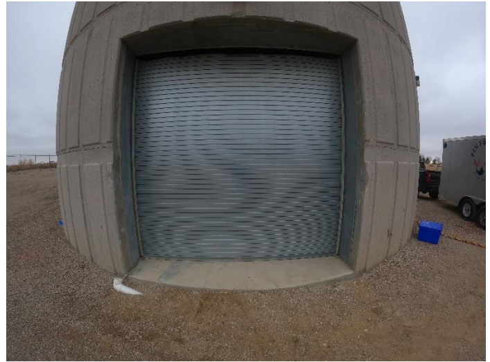
Exterior Conditions Excellent Condition, site well maintained and structure clear of vegetation.
